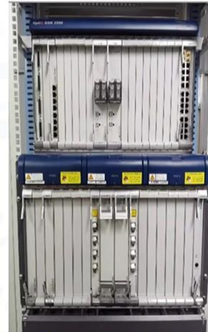
Optical Transmission System SDH Equipment Huawei OSN 3500
